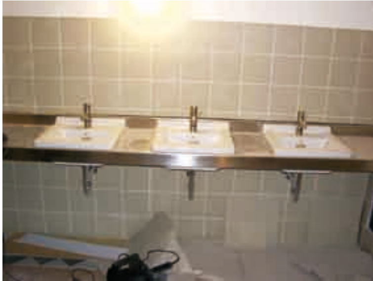
Figure 4: Ceramic sinks in an stainless steel washstand with vacuum connection at Burg Lenzen
