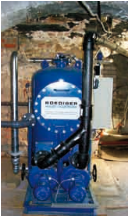
Figure 3: Basement vacuum station in the historical main building at Burg Lenzen, Germany
